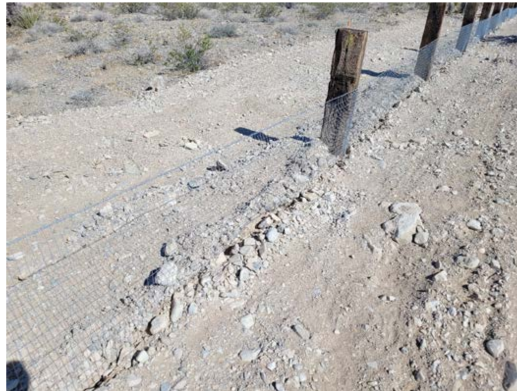
Twisted smooth wire at the top of the tortoise fence that was a design change from the original concept.
