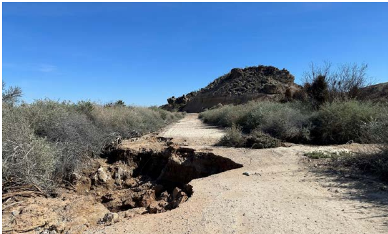
Storm damaged access road, Muddy River Reserve.
